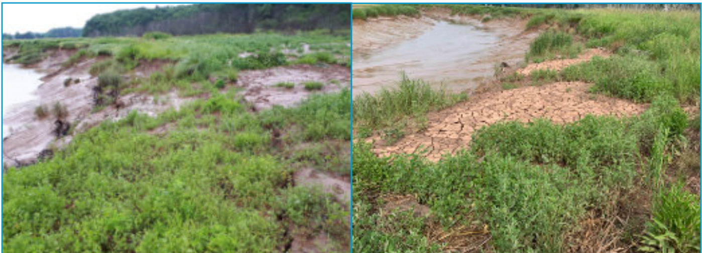
Hybrid rootwad living shoreline. Left: 2019 with erosion & slumping, Right: 2021 with reduced erosion & post adaptive management. PHOTOS: CBWES INC.
