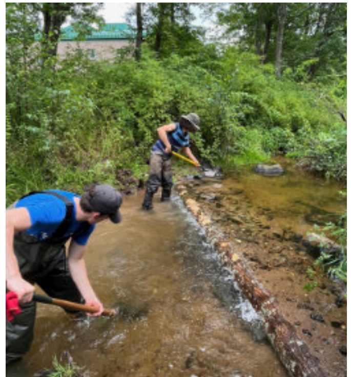
Harrison Basquill and Jonas Gow building up the rock ramp on one of the seven digger logs. PHOTO: WILL CHAPPLE.
