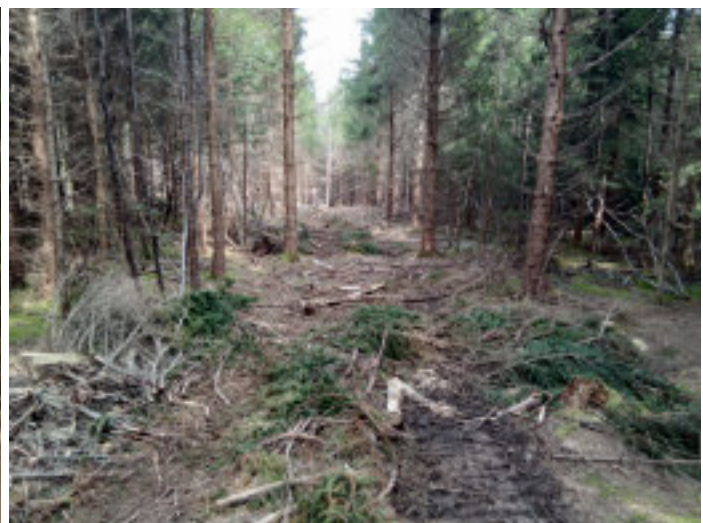
A forwarding trail was used to transport the logs out of the woods for roadside pick up.
